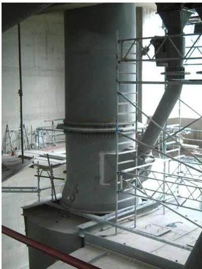
Installed A TEC Splash Box
