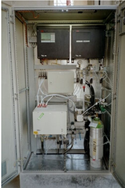
Gas treatment and analyzing cabinet
